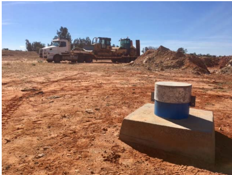
Figure 4. Installed Production Bore used to Commission the Pilot Solar Evaporation Pond Network
